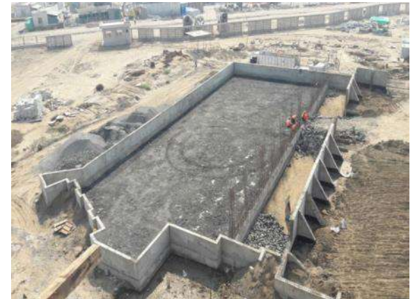
Reflecting pool – Rubble soiling
